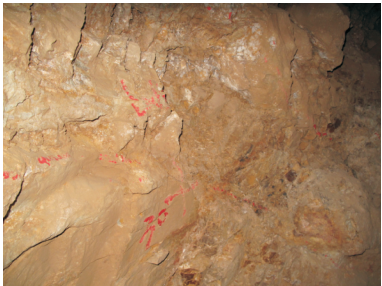
图 3 PD54 号平硐 30 m 处岩体呈碎裂-散体状 Fig. 3 Fragmented rock mass at 30 m of PD54
